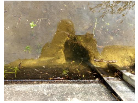
8 Leak hole at Virworthy spillway
