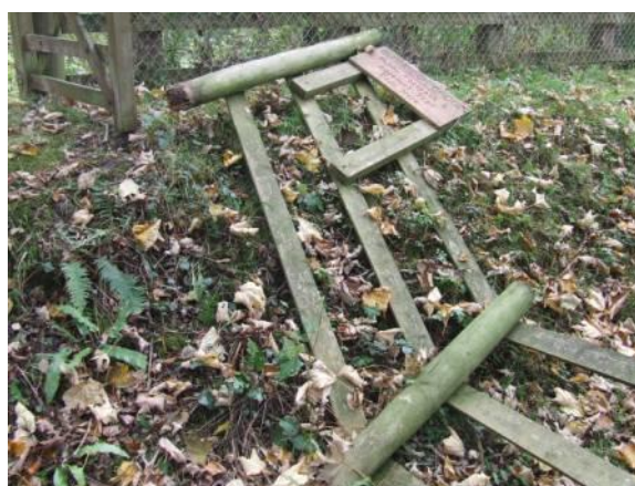
13 Rotted support posts
