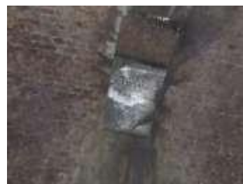
3 Water entry opening in roof
