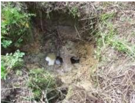
1 exposed rotten wood culvert
