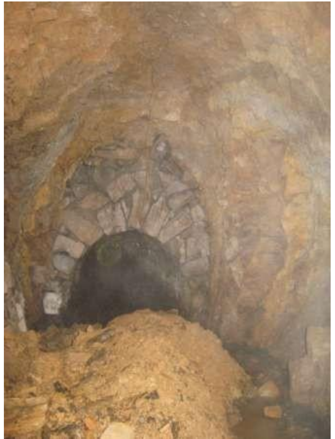
10 Roof fall material
