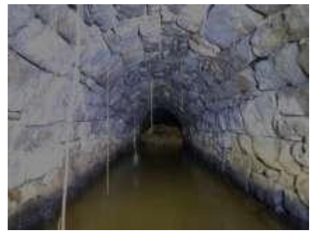
12 entrance lined tunnel looking into fallen soft ceiling
