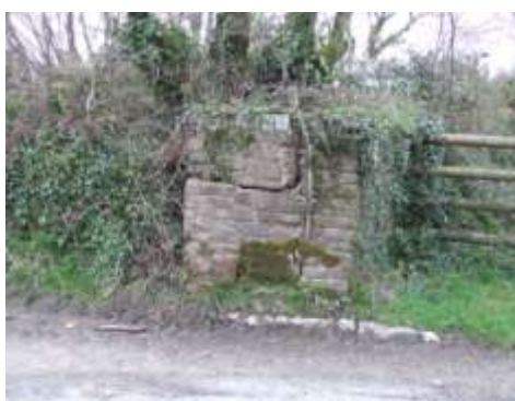
10.Puckland bridge damage
