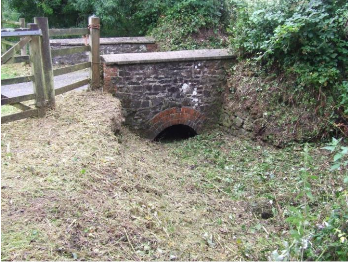
15.Dexbeer Bridge cleared
