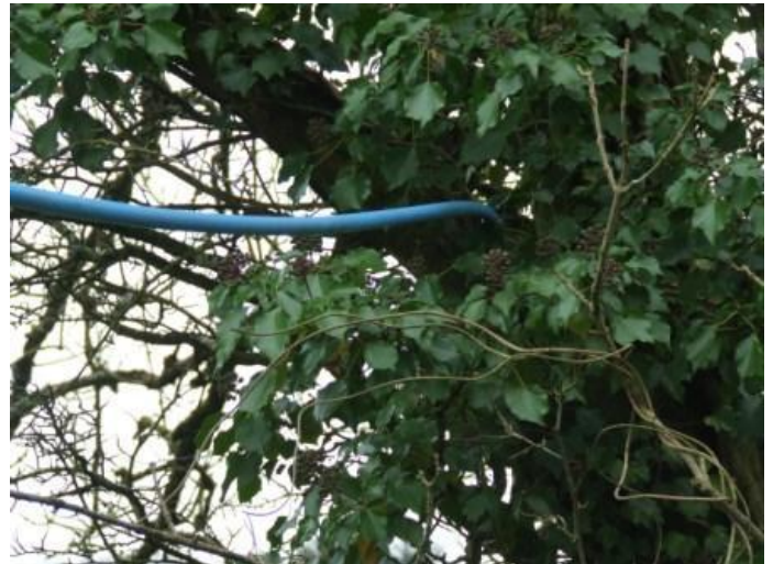
4 Gadlock water feed pipe through tree
