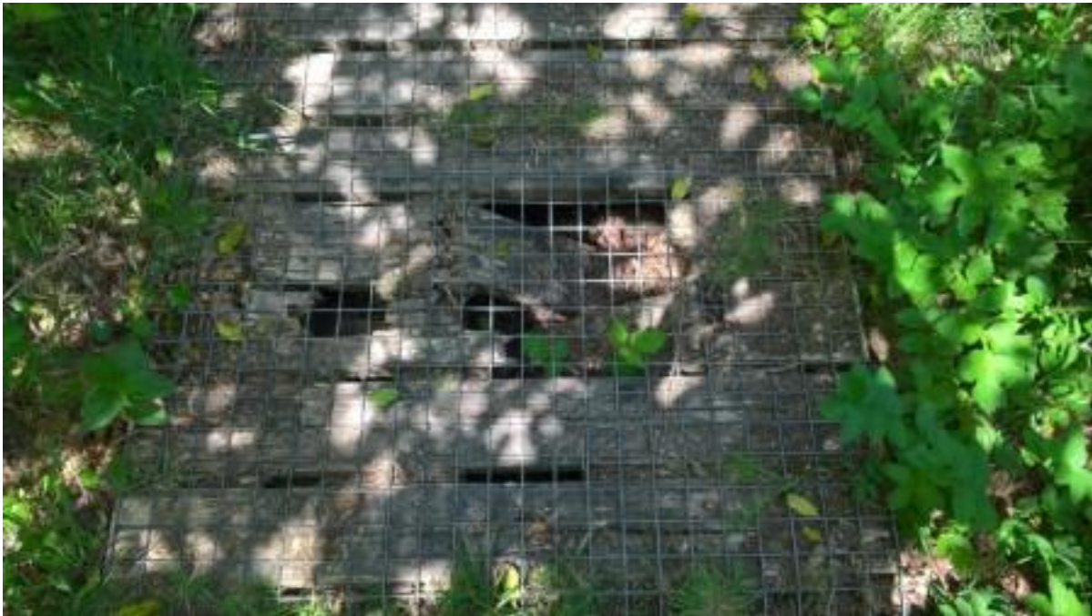
32 Bridge ramp damage at DNR
