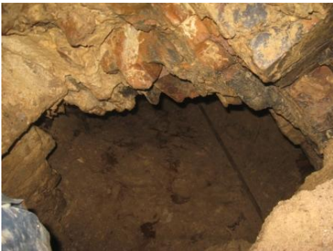
9 Remains of a collapsed arch
