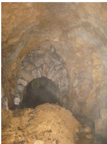
3 Roof fall material
